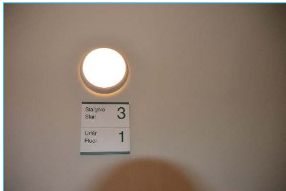
Figure 18. Light fitting directly above signage, glare
