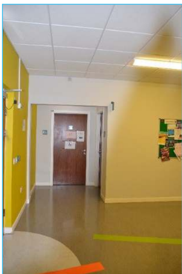
Figure 19. Accessible toilet locked and poor signage to all toilet facilities
