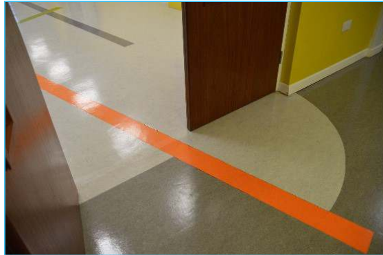
Figure 12. Contrasting floor pattern, in entrance and reception areas adds unnecessary visual clutter, could be misinterpreted as obstacles and changes in levels
