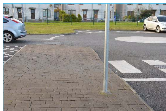
Figure 4. No blister paving at crossing point.
