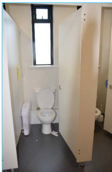
Figure 20. No ambulant disabled grab rails and lack of contrast
